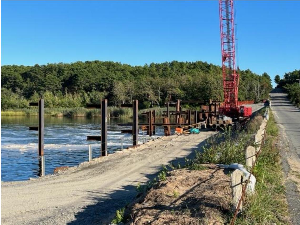
Work continues on the Herring River restoration project. Photo by Phyllis Bretholtz
